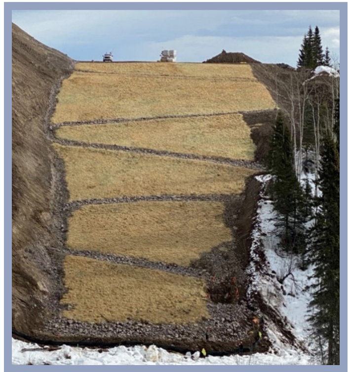
View of stripped ROW in preparation for open cut, temporary ESC measures (straw, cross ditches, rock armour and seeding)
