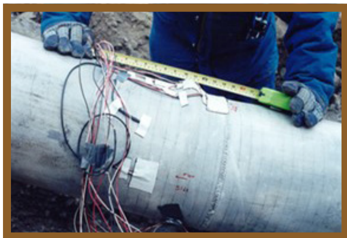
Figure 2. Compressive wrinkle in an NPS 12 (323mm outside diameter) pipeline induced by slope movement
