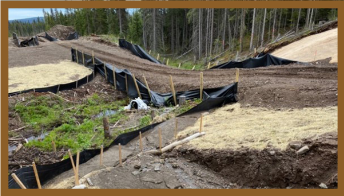
Example of poorly maintained BMPs and possibly the wrong BMPs chosen to direct water off the ROW before the bottom of the slopes
