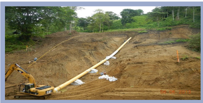
Figure 5. Pipeline and slope remediation after a slope movement induced pipeline rupture that leaked crude oil into an adjacent stream.
