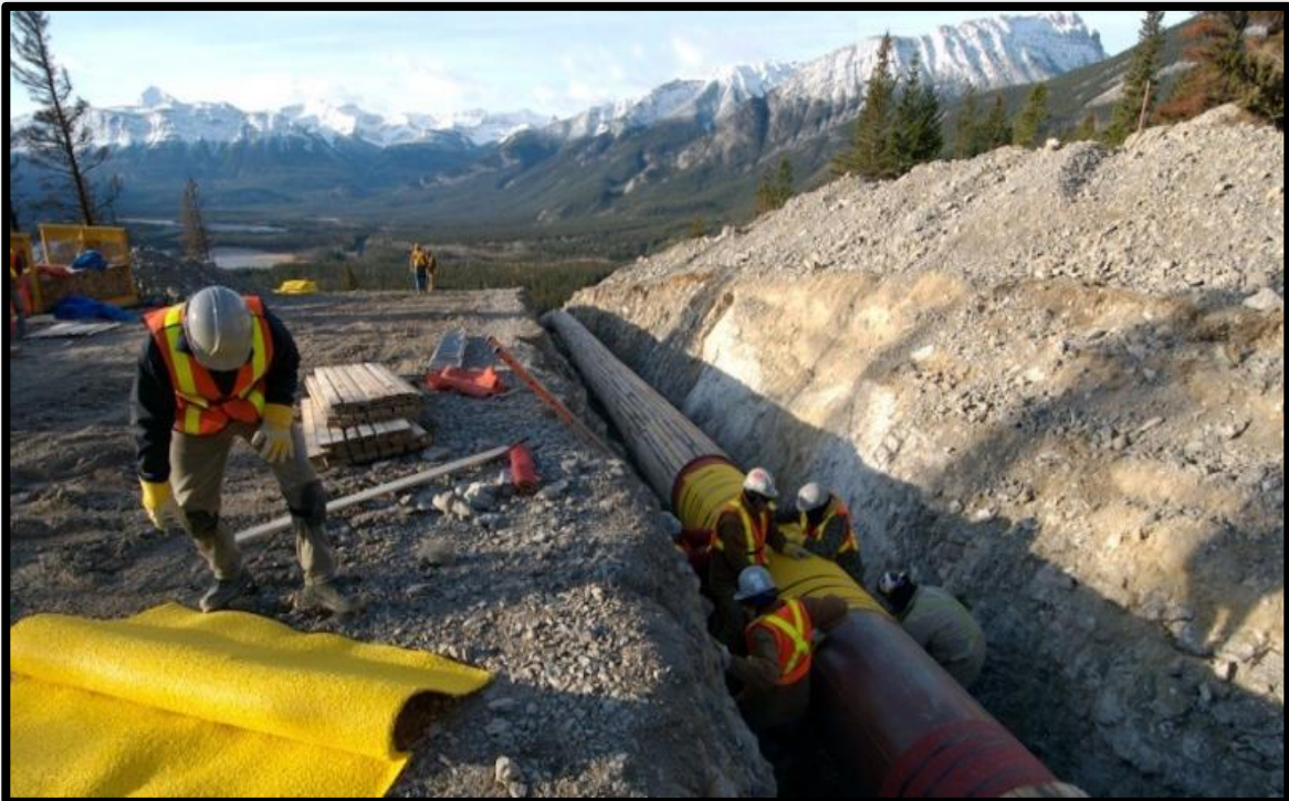
Pipeline workers are installing protection around a pipe section when lowered in to a rocky trench
