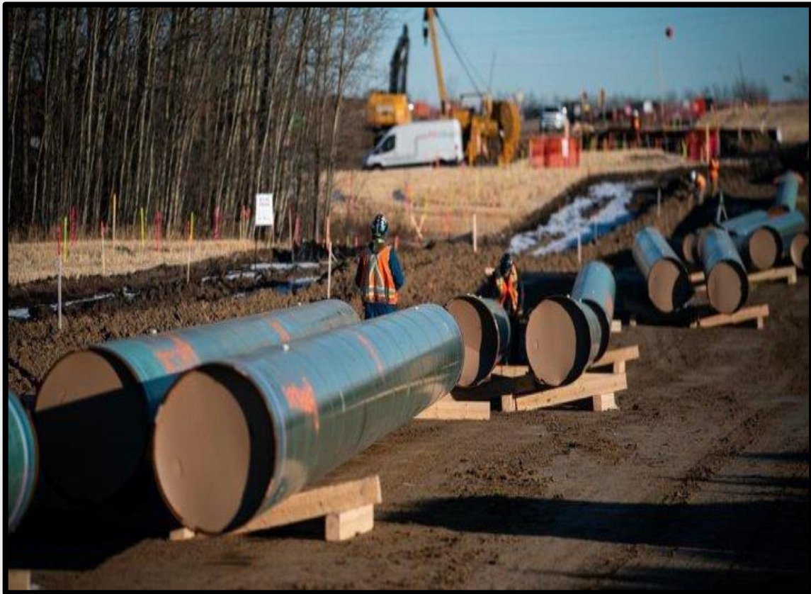
Pipeline contractor has strung pipe joints that have cardboard end-caps on them.
