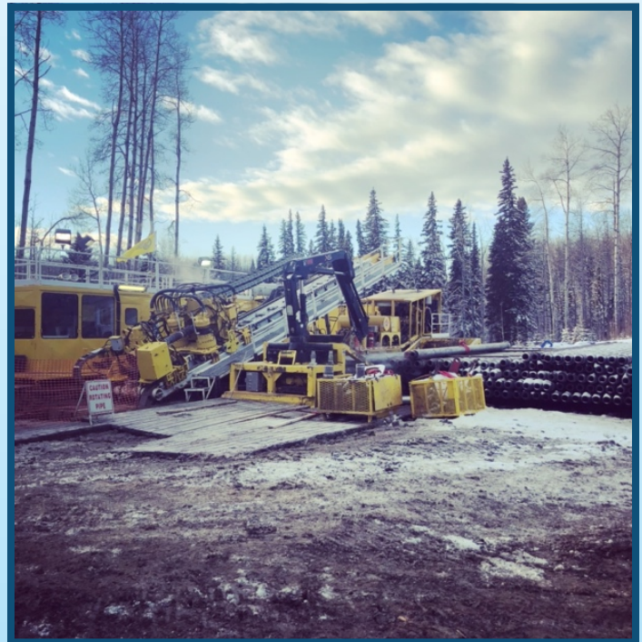
Horizontal directional drill piloting hole across a large permanent fish bearing watercourse, trenchless method
